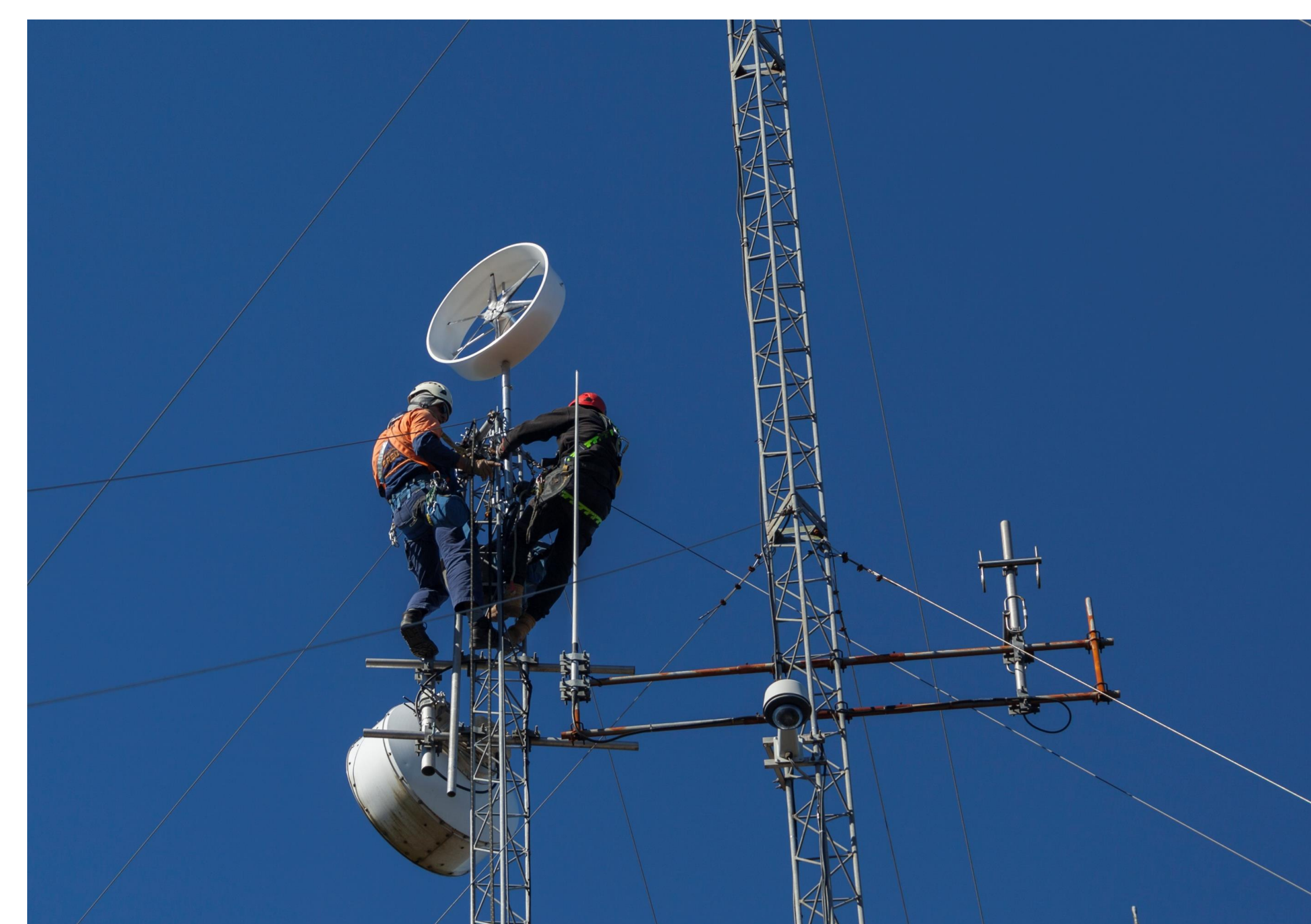
Figure 2: Installation at a telecommunication site.
